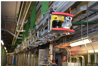
Train Inspection Monorail - TIM
